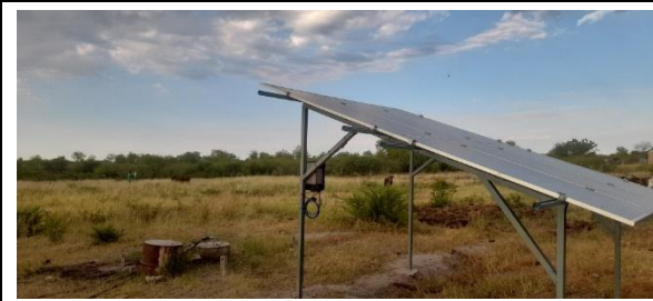
Photo 4-19 Solar panel used at boreholes
