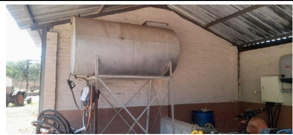
Photo 4-20 Fuel storage tanks
