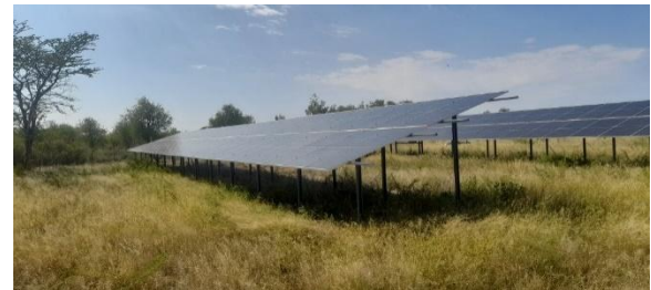
Photo 4-22 Photovoltaic solar system
