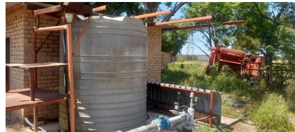
Photo 4-12 Fertiliser mixing tank
