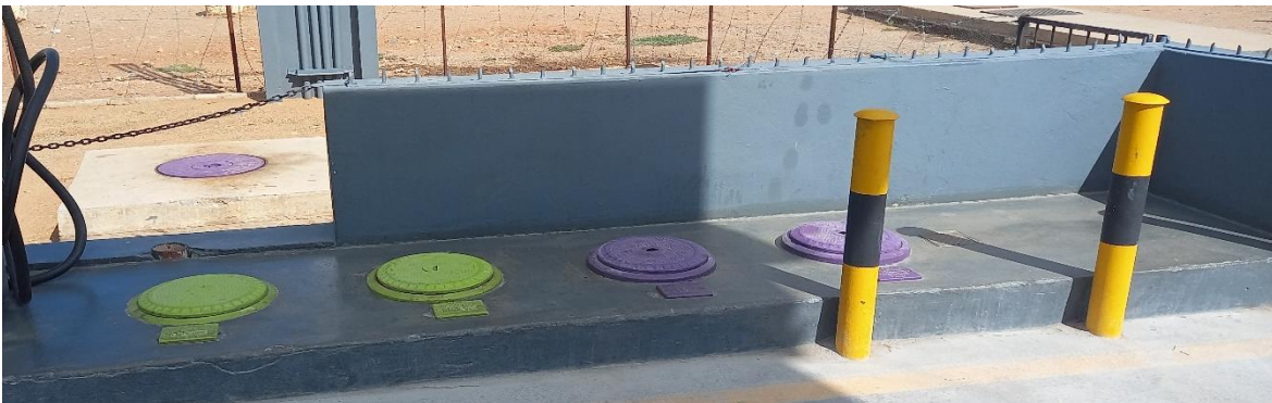
Figure 9: Fuel Receiving Points from Road Tankers
