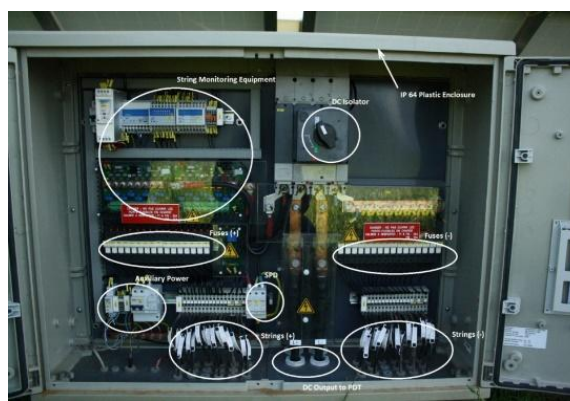
Photo 5-4 Typical enclosure components
