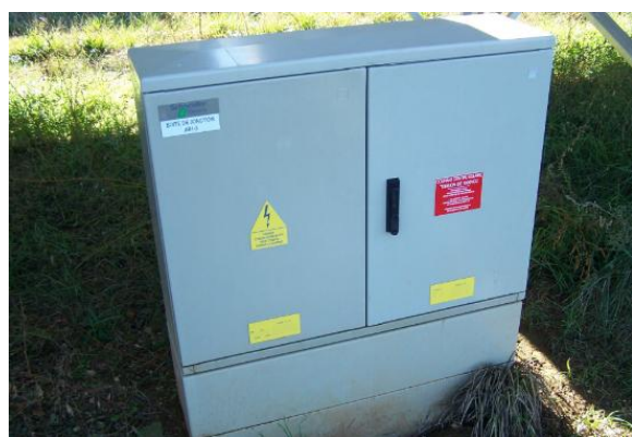
Photo 5-3 Typical array enclosure
