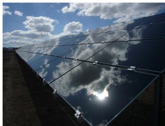
Photo 5-2 Typical PV array
