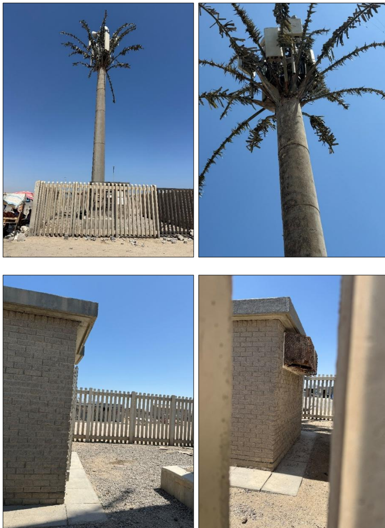
Figure 2-1: Photos of the current (dilapidated) status of the DRC tower and associated supporting infrastructure (accessories)
