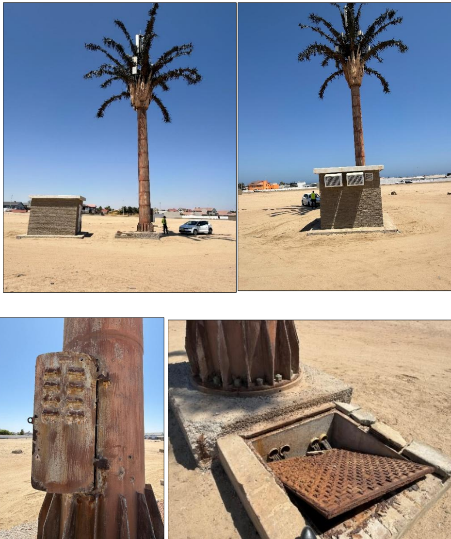
Figure 2-1: Photos of the current (dilapidated) status of the Ocean View tower and associated supporting infrastructure (accessories)
