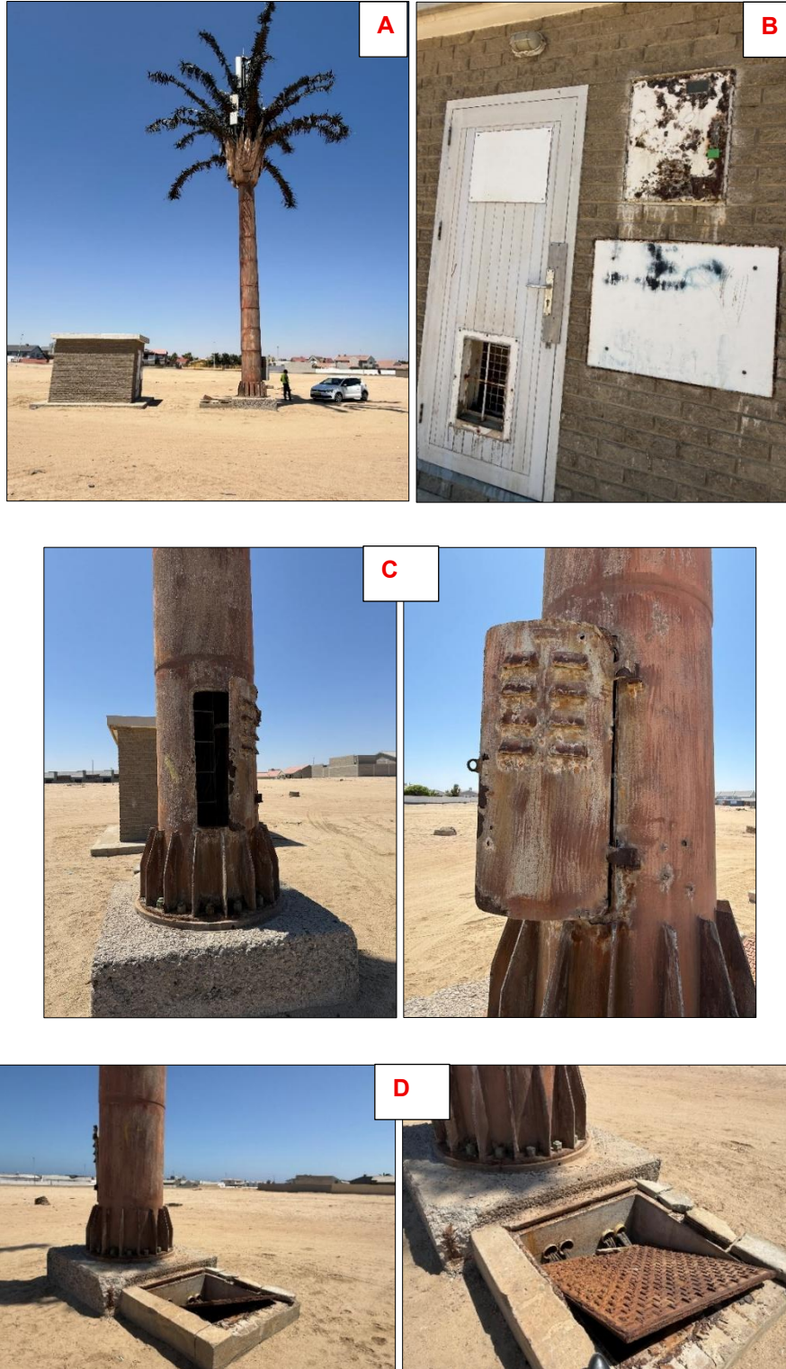
Figure 1-3: Photos of the current (dilapidated) status of the Ocean View tower: A- The monopole tower with artificial leaves/branches and rectangular antenna boxes and support infrastructure (cabinet); B- Dilapidated front of the tower equipment cabinet; C & D- Dilapidated tower base foundation equipment
