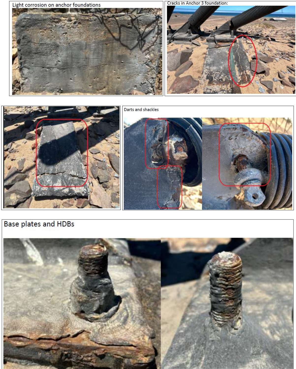
Figure 1-3: The Condition of the Terrace Bay tower anchors in February 2026 (source: Klein and Shishiveni, 2026)
