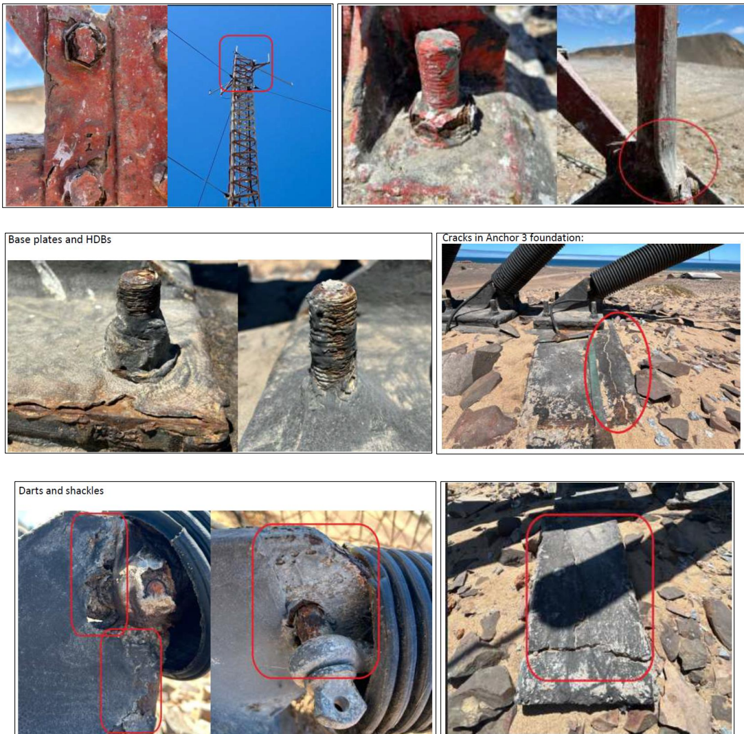
Figure 2-1: Photos of the current (dilapidated) status of the Terrace Bay tower and associated supporting infrastructure (accessories) (source: Klein and Shishiveni, 2026)
