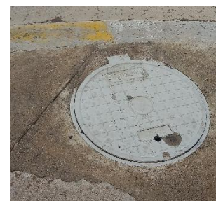
Figure 14: Paratus fibre-optic network manhole cover
