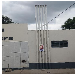
Figure 7: Vent pipes from the tanks
