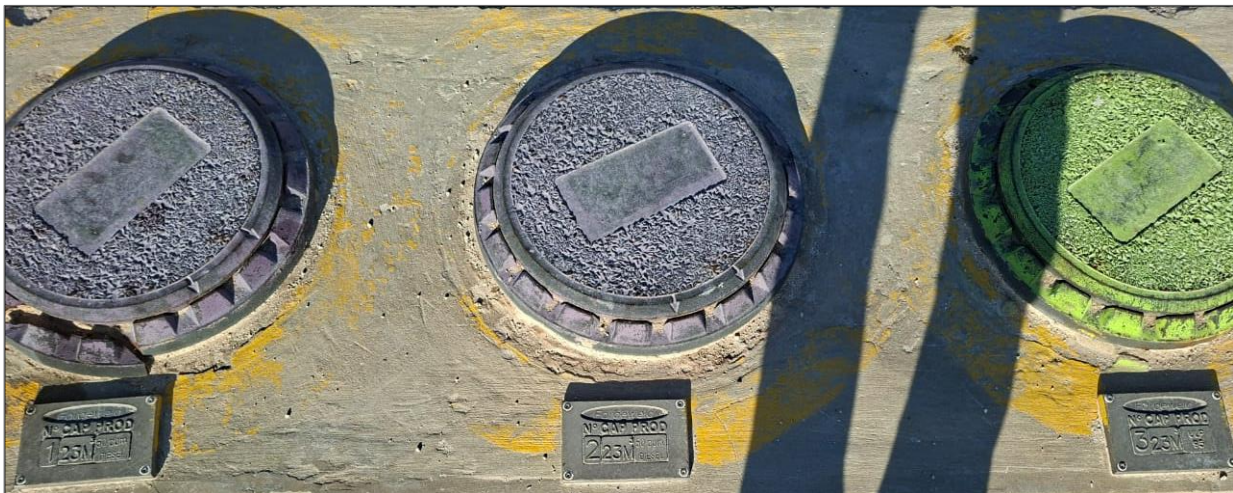
Figure 2: Underground storage tanks at Omakange service station.
