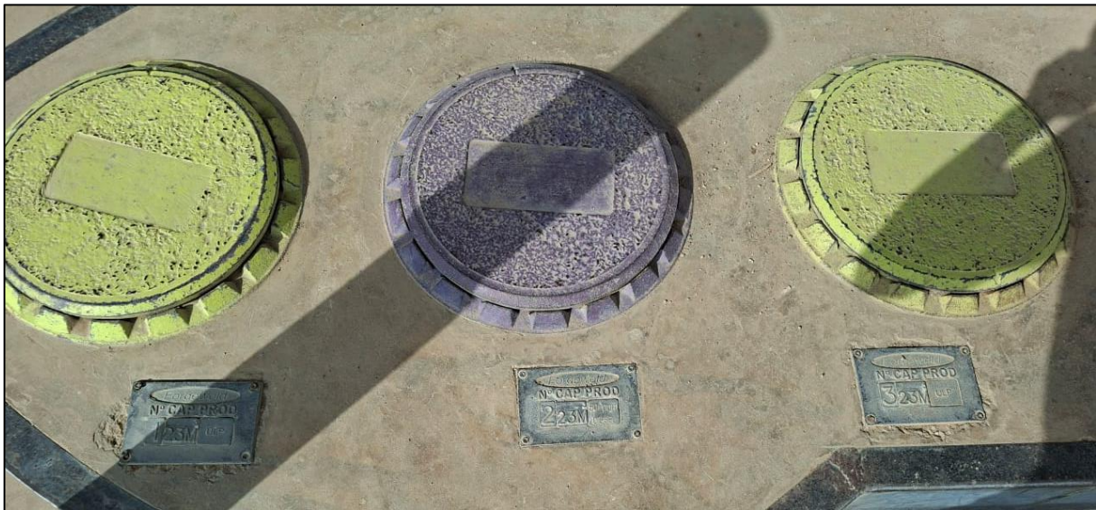
Figure 2: Underground storage tanks at Ohakane service station.
