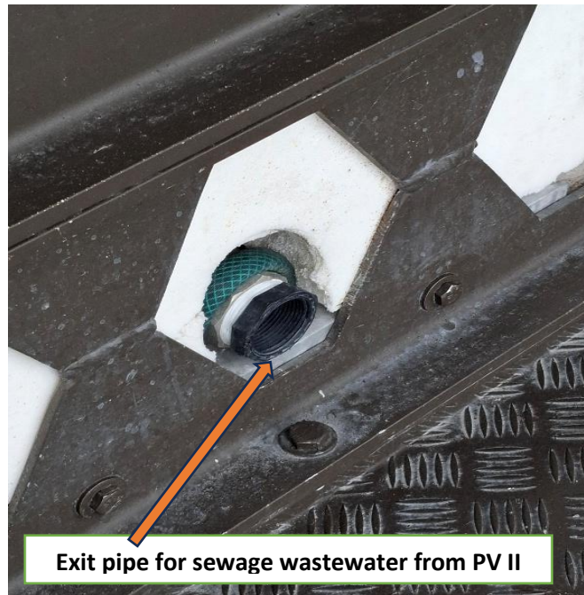
Figure 11: Outlet pipe for sewage wastewater connected to transport boat during emptying of septic tanks (rear of the PV)
