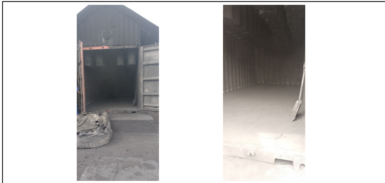
d) One of the dust collectors on site which is well cleaned
