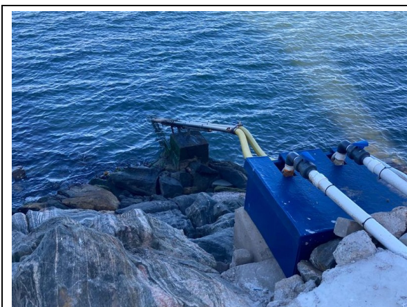
Photo 4-11 Seawater abstraction point
