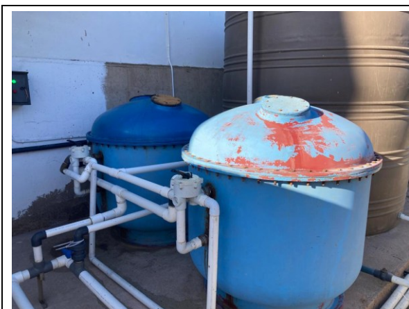
Photo 4-9 Sand filters used for water filtration
