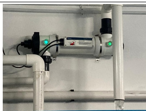
Photo 4-10 Ultraviolet disinfection unit installed in the water supply line
