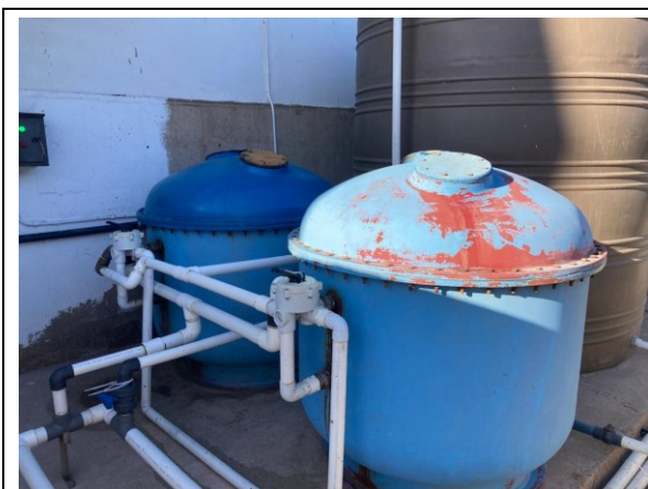
Photo 4-9 Sand filters used for water filtration
