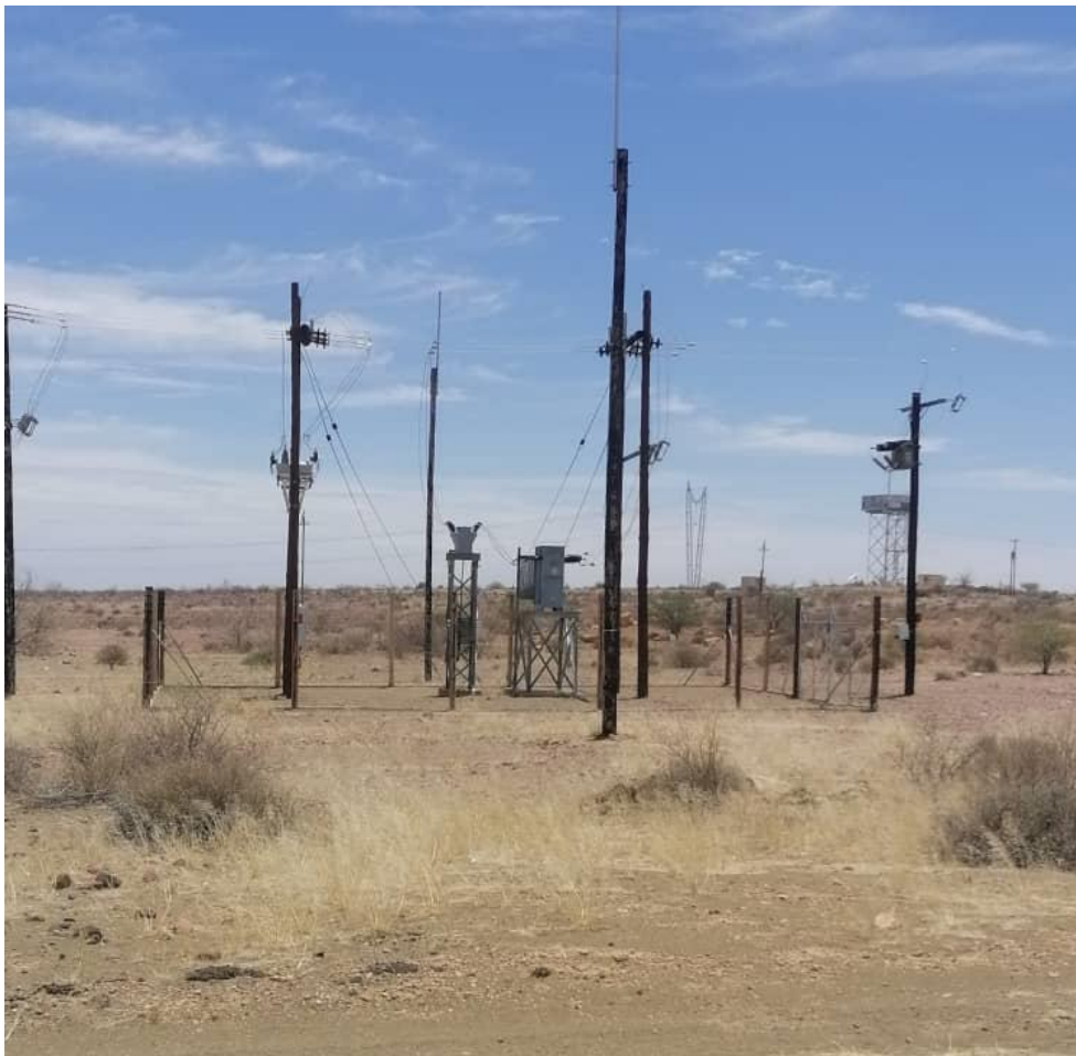
Figure 6: Sub-station and powerlines opposite the proposed site
