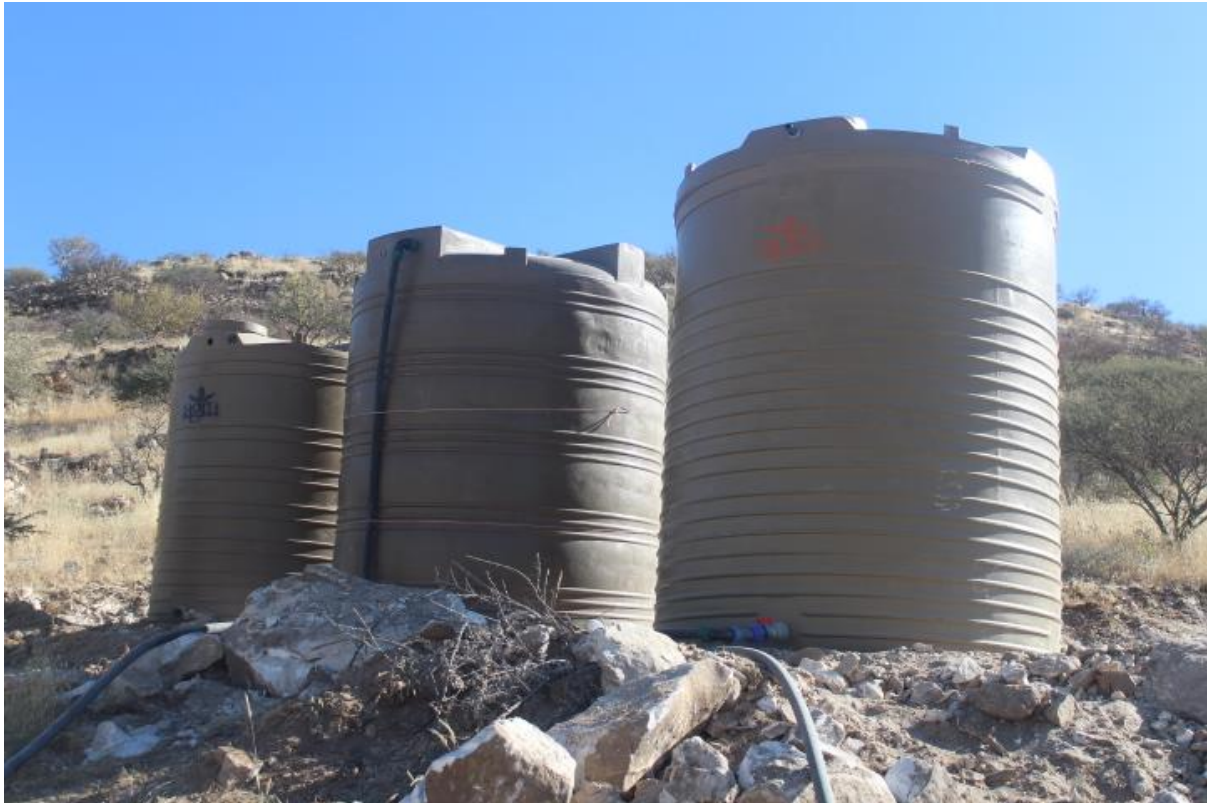
Figure 5: The waters tank that will be used for water storage during the operation of the mine.
