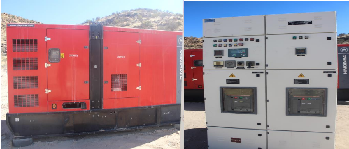
Figure 4: A 420 Volts generator that will supply power at the site.
