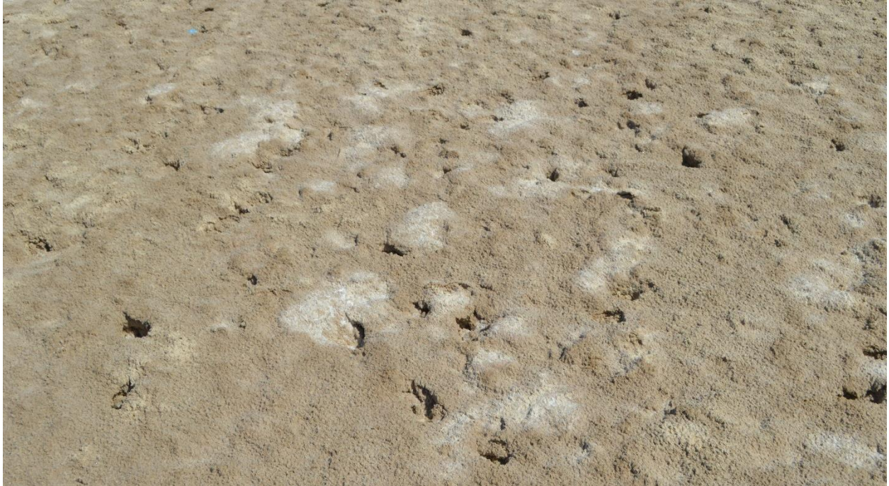
Figure 18: Soft and unstable ground
