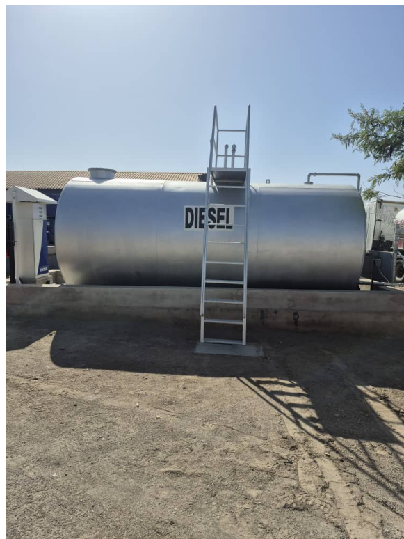
Photo 4-1 Diesel storage tank in bund area
