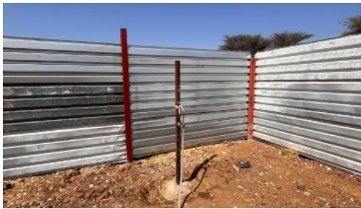
Water Tap on site
