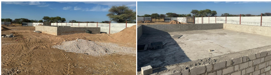
Figure 5. Fuel Tank Platform and 110% spill containment wall
