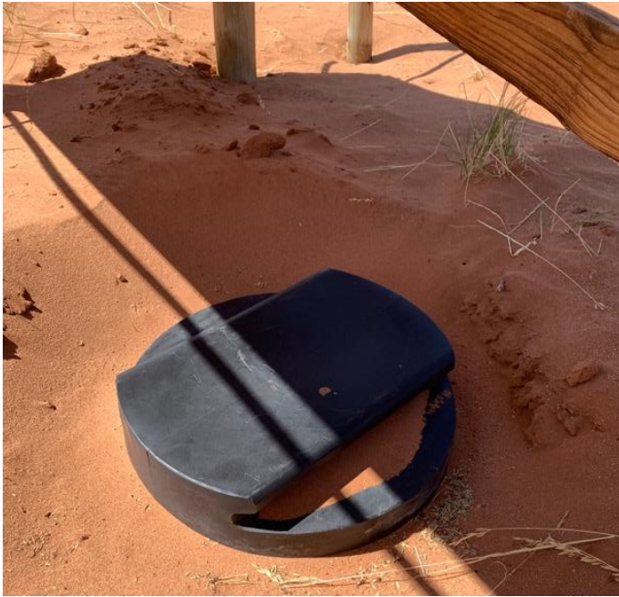
Figure 14. Campsite sewage goes into a septic tank and then to a French drain.
