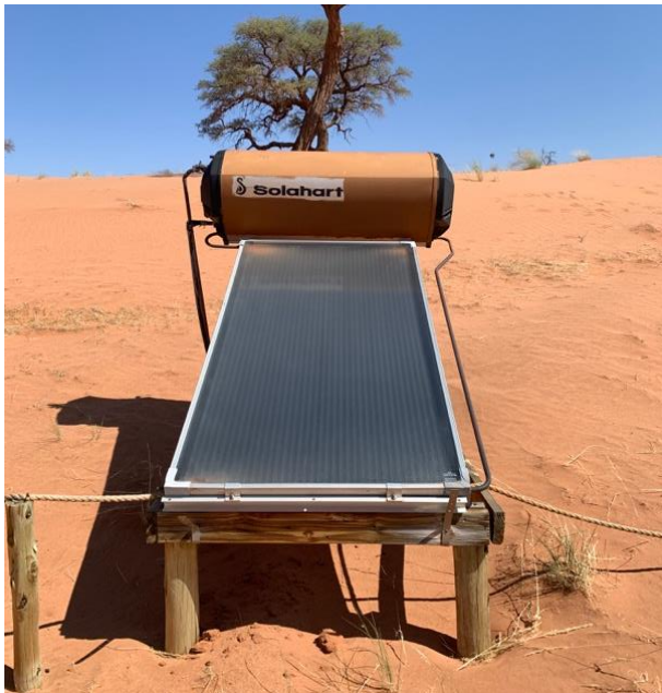
Figure 13. Solar geysers at the campsites.
