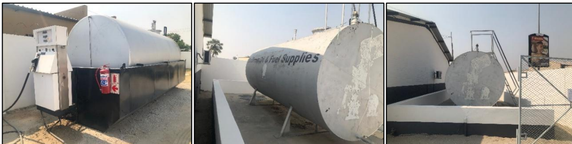
Figure 5: Tanks present on site
