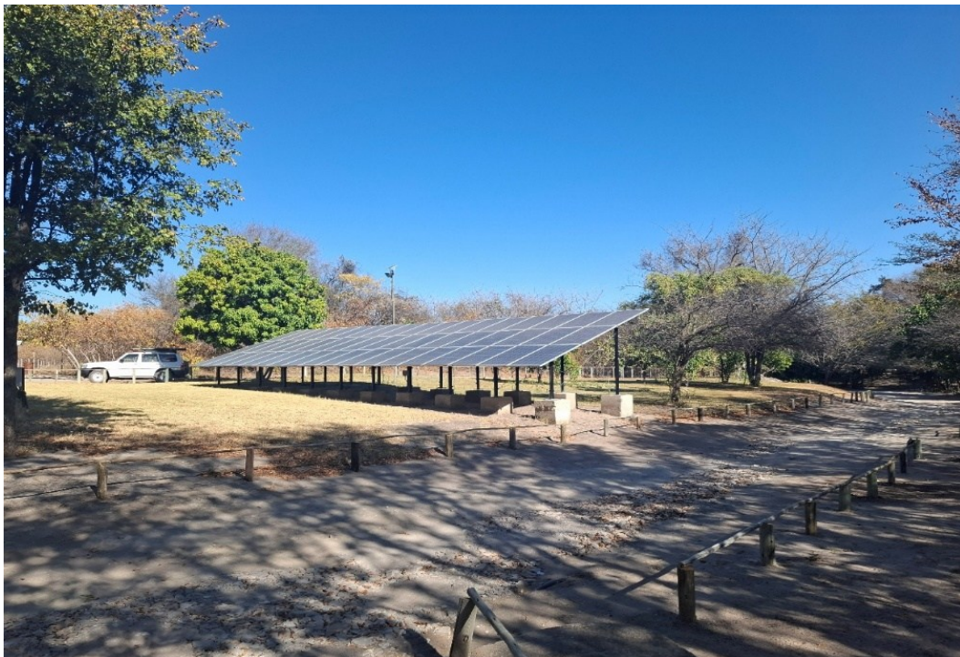
Figure 6: Solar panels at Camp Kwando that generate 95% of all energy requirements (E Klingelhoefter).
