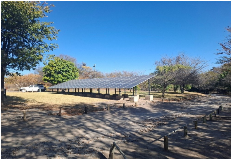
Figure 6: Solar panels at Camp Kwando that generate 95% of all energy requirements (E Klingelhoefter).
