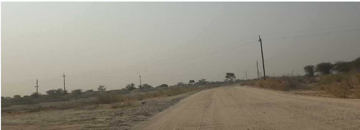
Figure 8: Project Site - Northern view with heaps of road materials upgrade to the left
