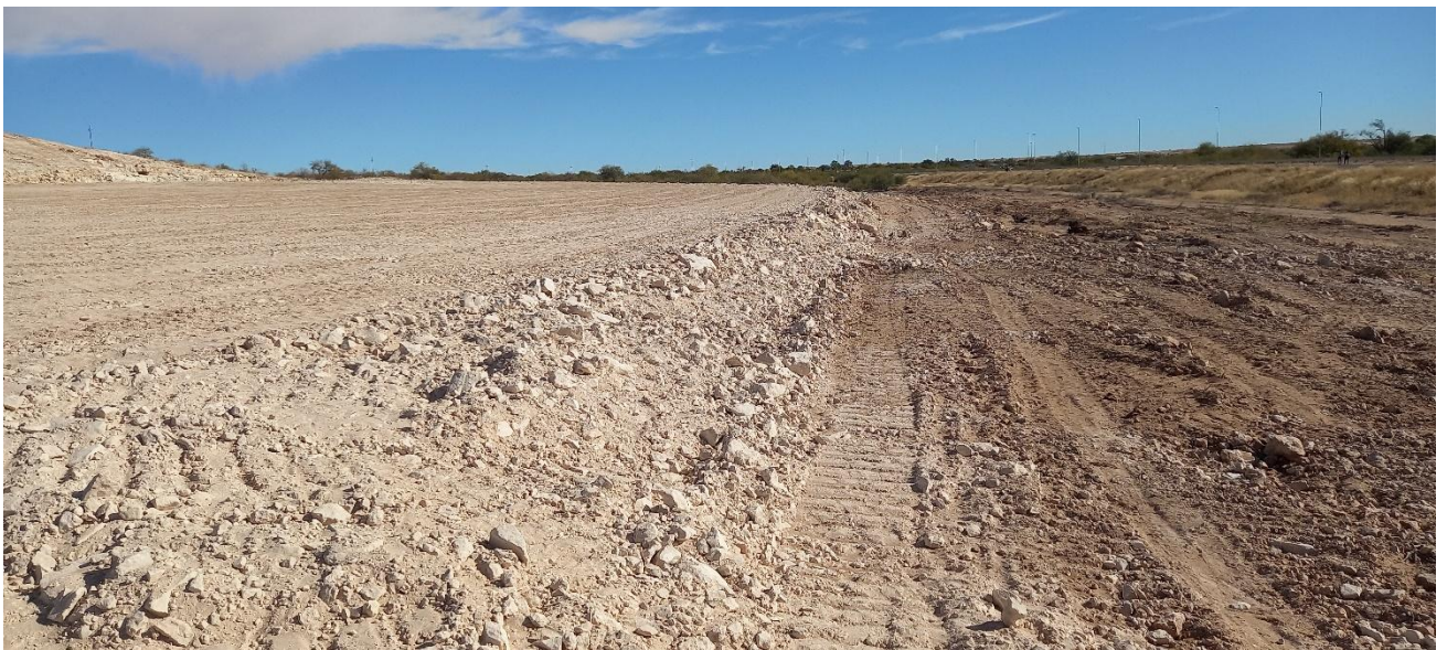
Figure 5: Site Preparation for the Shopping Complex Development with Backfilling and Levelling Underway. Note Height of Filling
