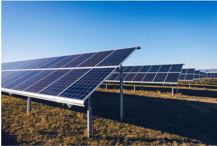
Figure 8: Heightened Solar Panels (For illustrative purposes only)
