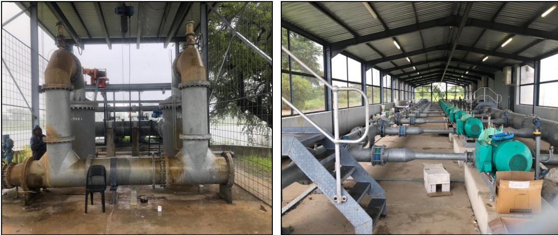
Figure 10: The main and booster pumpstation
