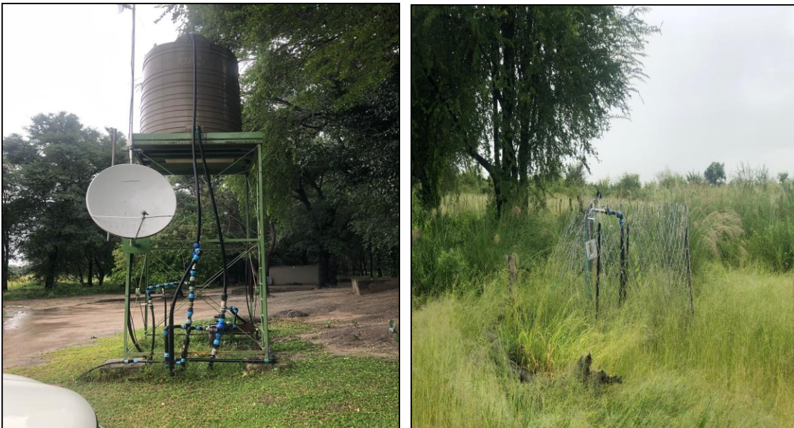
Figure 9: Water storage tank and water connection
