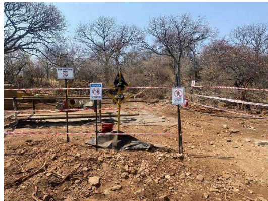
Photo 4-9 Safety signage and demarcation of restricted areas at drill site
