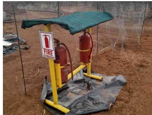
Photo 4-10 Firefighting equipment at drill site
