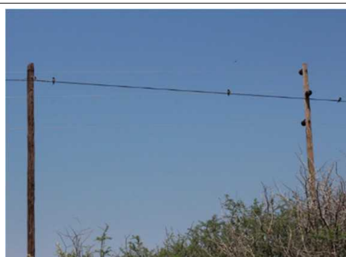
Photo 7-18 Electricity transmission lines
