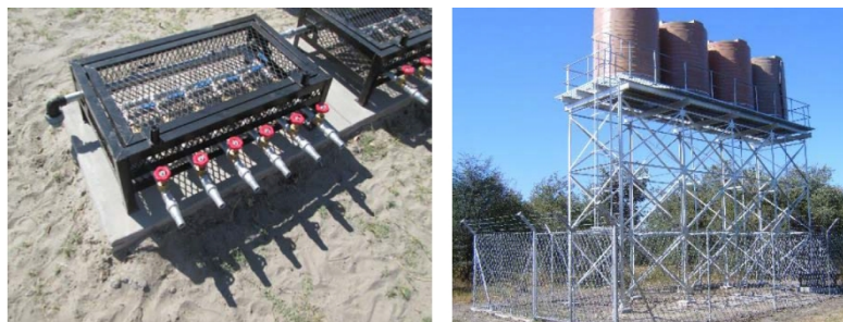
Figure 4: Manifolds (water meters) and elevated water tanks at Phase 2 (LCE, 2022).
