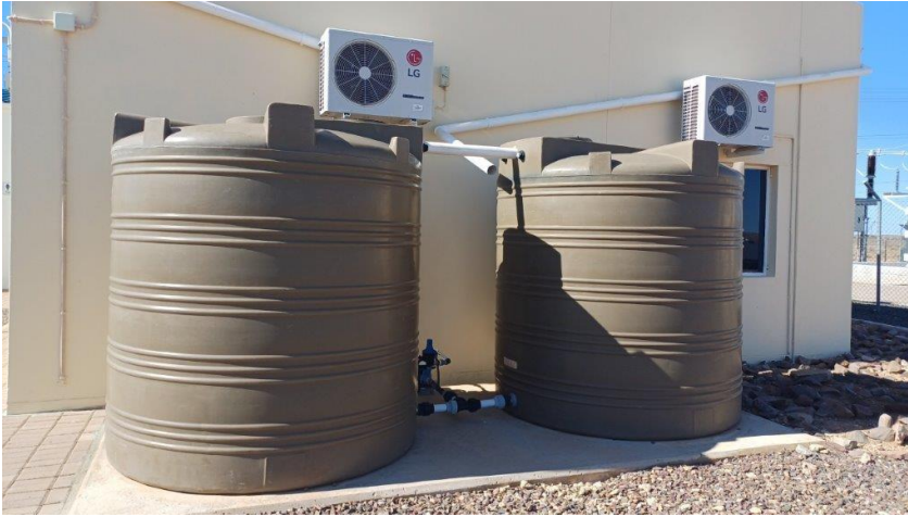
Photo 18 – View of potable water tanks at site office.
