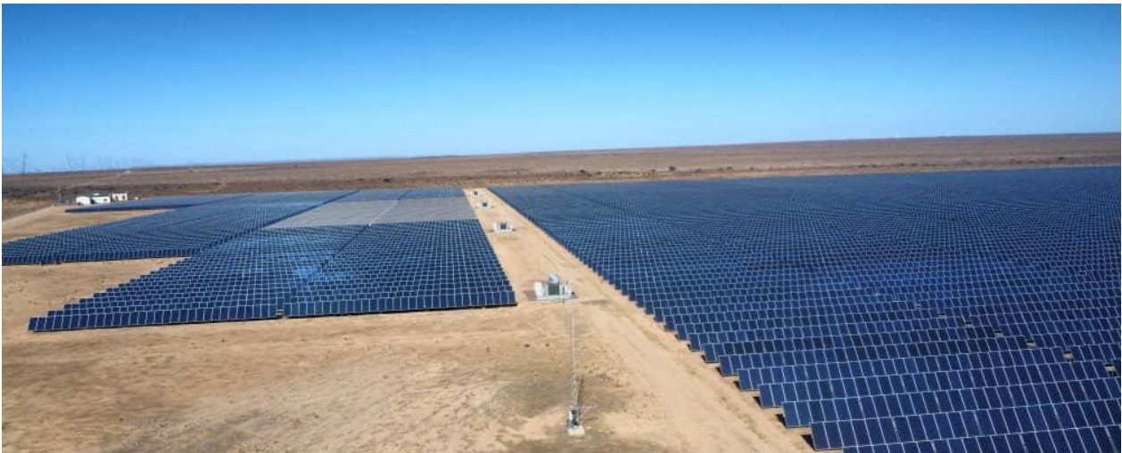
Figure 2: Illustrate the typical installation of solar panel field, similar to which DanAon Energy envisage to install
