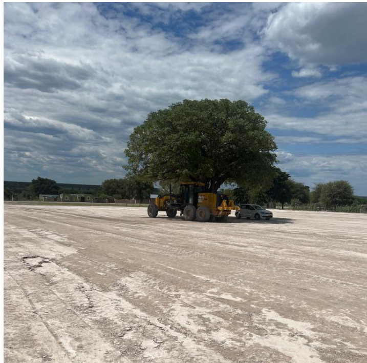
Figure 14: Illustrates the clearing of land for the proposed site in Gcamade Mbunza, Kavango West Region.
