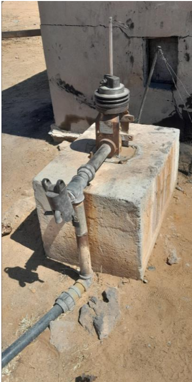
Figure 2-7: Old equipped non-functional borehole in the settlement
