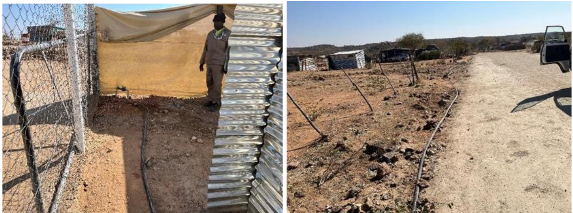
Figure 2-5: Installed prepaid water meter and water pipes in Ourab
