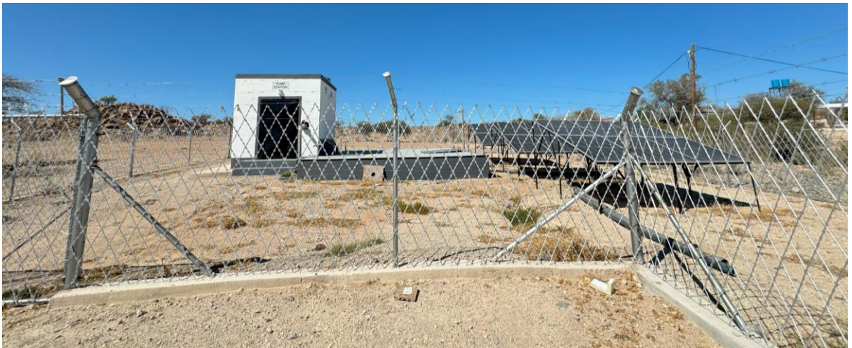
Figure 2-4: Solar Panels Installed for Bulk Water storage facility
