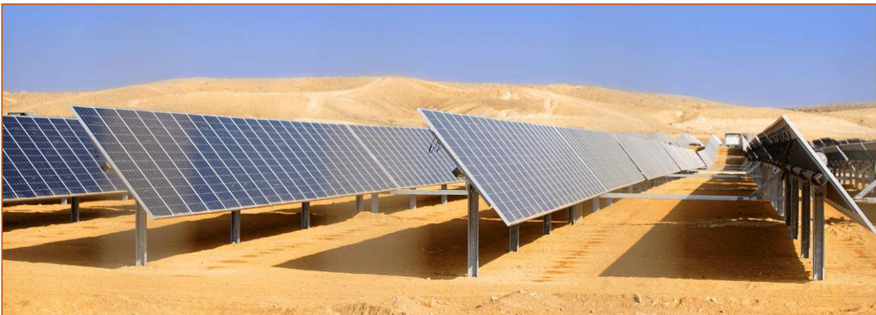
Figure 2: Illustrate the typical installation of solar panel filed, similar to which DanRe Sun envisage to install
