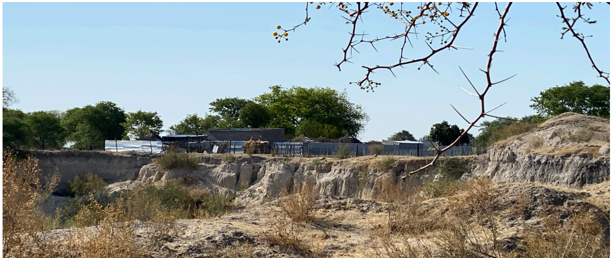
Figure 8.9: Un-rehabilitated, Sand mining borrow can be very dangerous to people and livestock, Okaku constituency (TEC, 2022)
